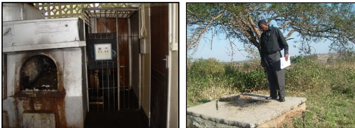
Figure 3-23 The incinerator and a lined pit at a hospital
